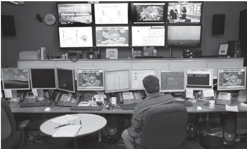
FIGURE 7.5 Internet-based supervisory control and data acquisition systems can save money and make systems easier to administer, but they also carry security risks. (© p77/ZUMA Press/Newscom)
